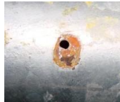
Galvanized Schedule 10 after only 18 months
